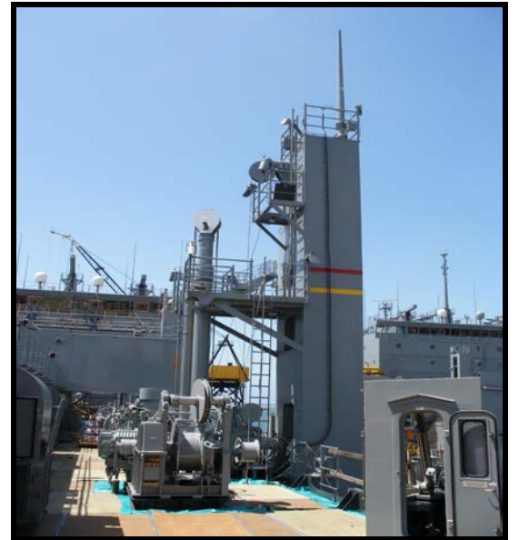
"UNREP" Tensioner Installed on T-AKE Vessel
