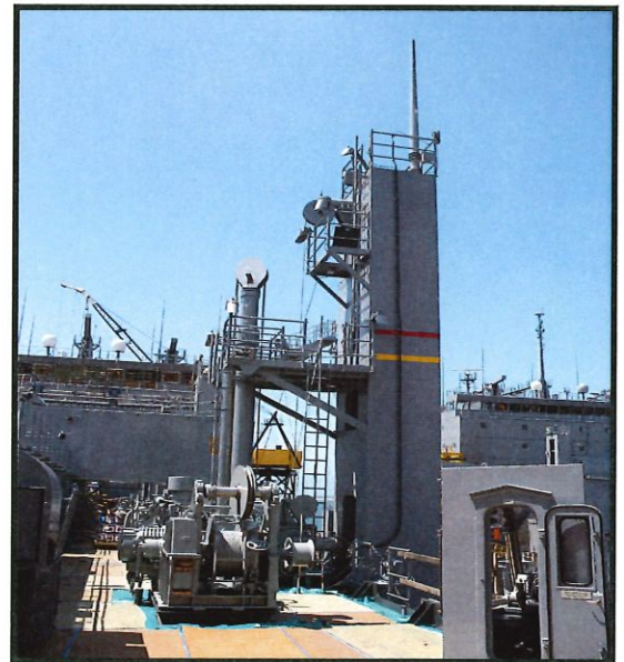
"UNREP" Tensioner Installed on T-AKE Vessel
